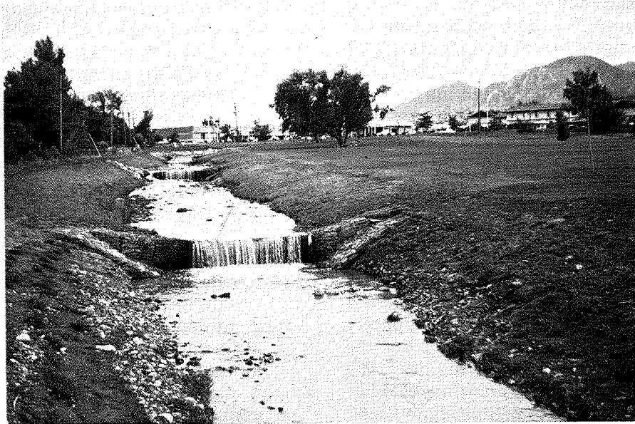
a. check dams across a stream, through an urban area in Rocky Mountain foothills
