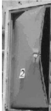
FIGURE 10.21: Conventional Hollow Metal Door Damage Under Low Blast Load
