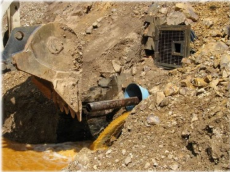
Gold King Level 7 Old Portal with well-point installed through the drain pipe. This point may be re-opened in a future project to help stabilize the mine drainage and prevent future increases in mine pool level.
