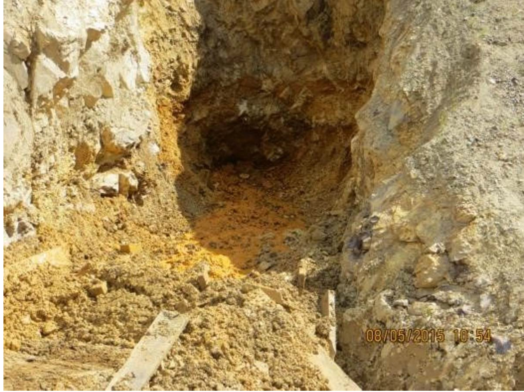
Figure 51.—Photograph of the uncontrolled flow taken at 10:54 a.m. on August 5, 2015. In 3 minutes, the flow progressed from a vertical spurt of water to the flow erosion evident in this photograph. The EPA OSC then made a decision to evacuate the portal opening to safeguard personnel onsite. A few moments later the flow erupted in an uncontrolled release (photograph from EPA project files).
