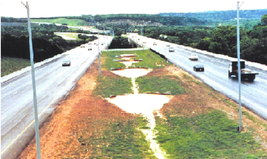
Figure 3.1 - Silt fences in series, on a relatively flat slope, pool water and decrease its velocity.
