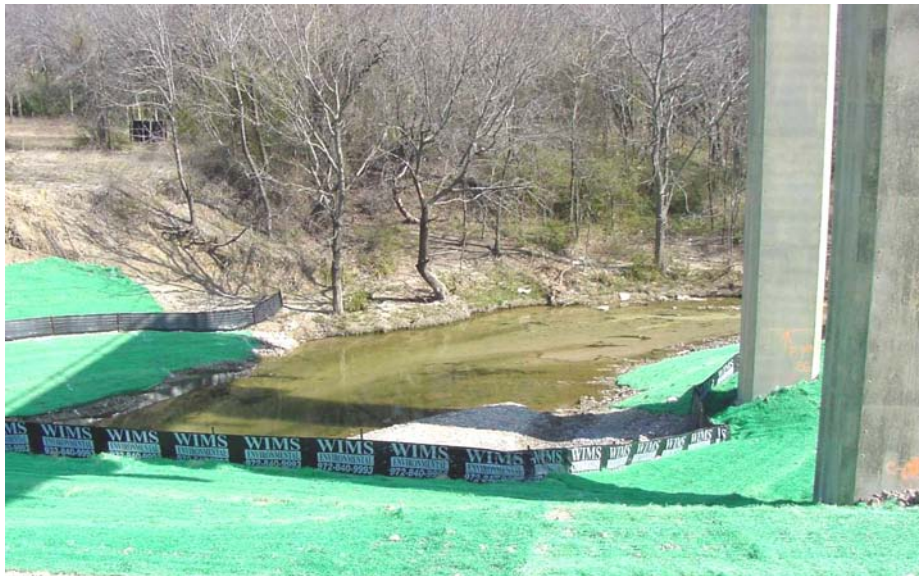
Figure 4.5 – Soil retention blankets used, in conjunction with silt fence, to stabilize a slope.
