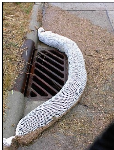
Figure 16. Temporary Erosion-Control Devices
