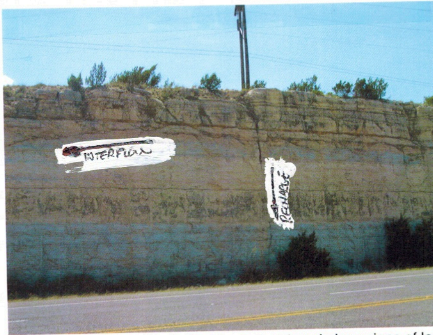
Figure 4.14. Photograph of feature in limestone showing obvious signs of large-scale water intake. Photograph taken by the author, US 277 in Schleicher County, Texas.
