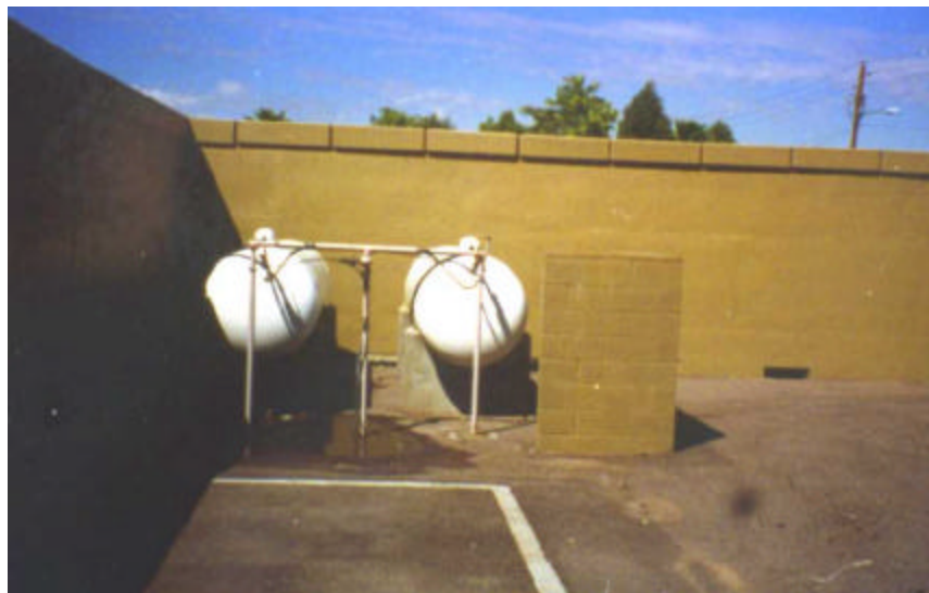
Figure 11-1. Liquid propane tanks for pump station power
