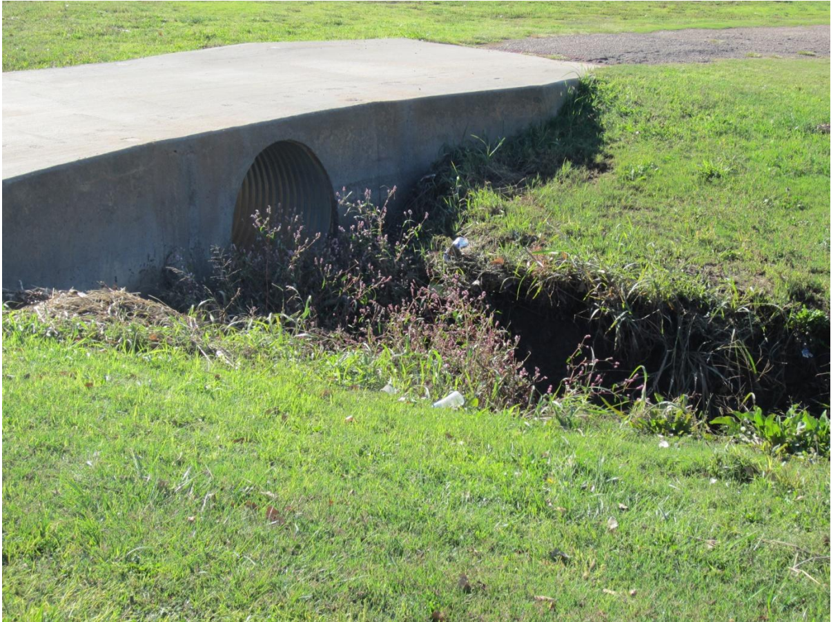
Figure #. View of the downstream side and top of the second culvert.
