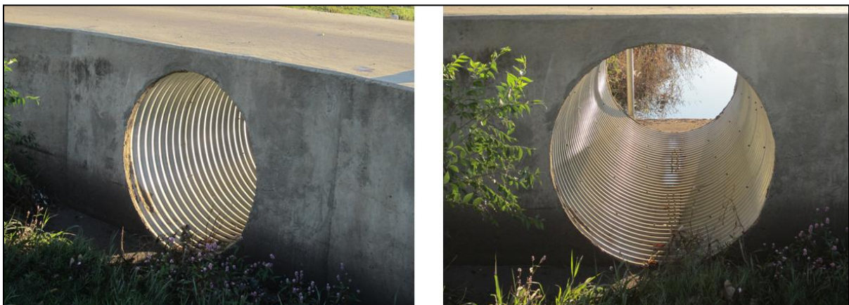
Figure #. View of the upstream culvert entrance and the corrugated metal culvert.
