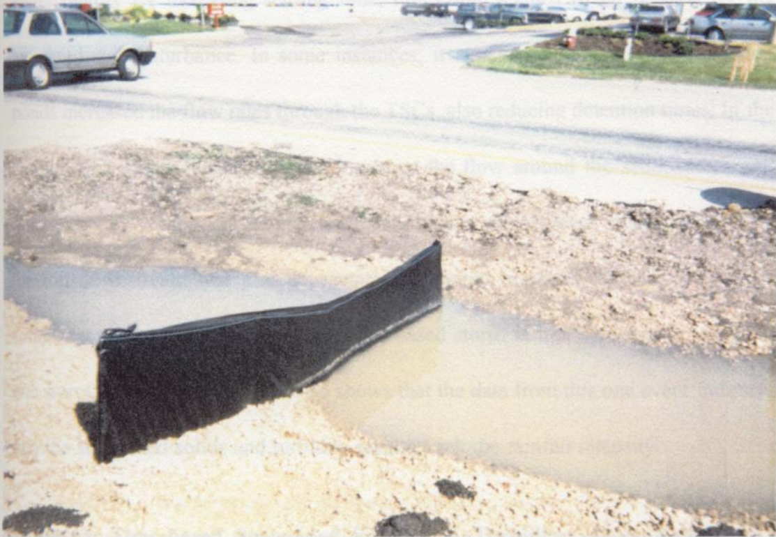
Figure 11: Sediment Control Fence with Runoff Flow around End of Fence Flowing onto Devegetated Area
