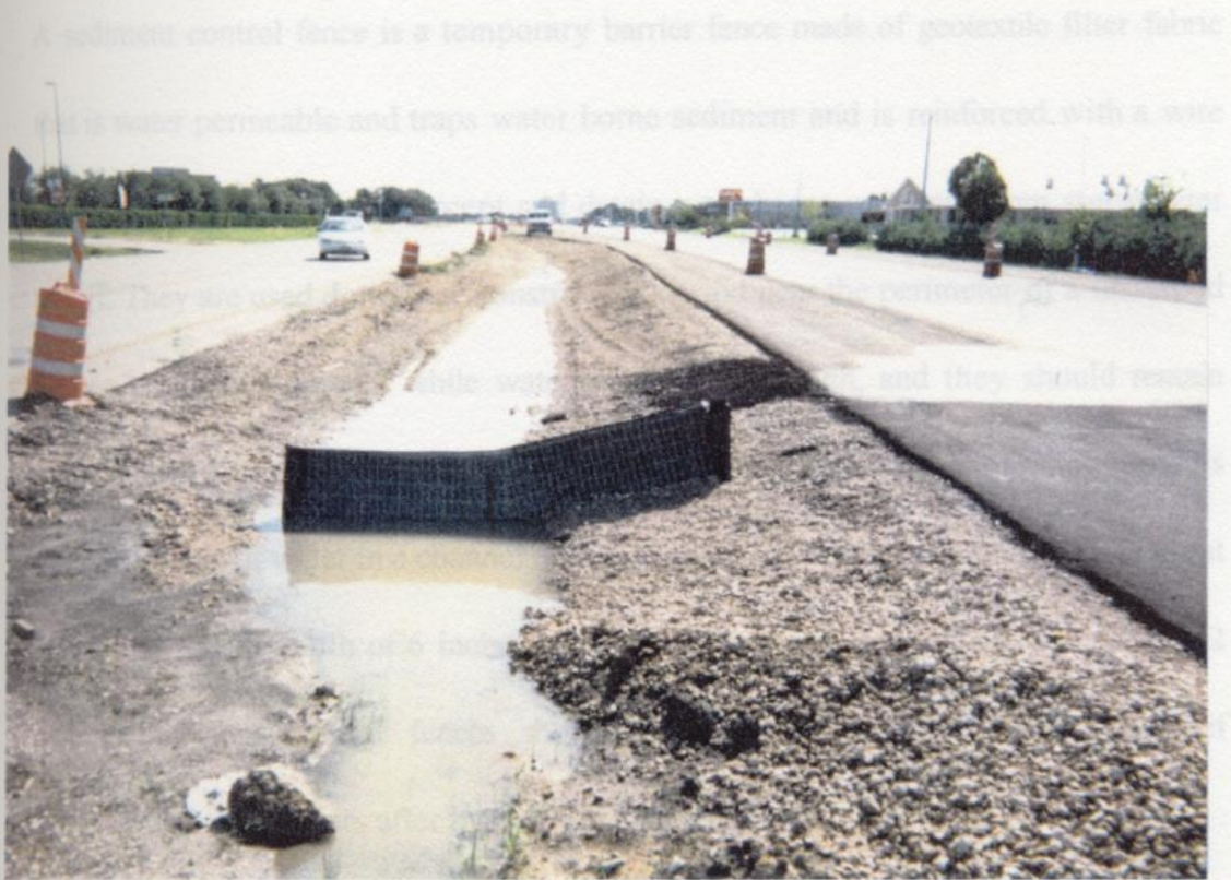
Figure 5: Sediment Control Fence TSC-2
