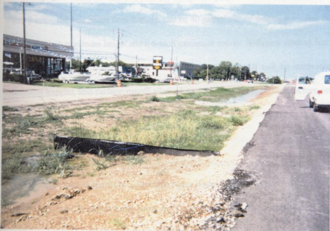
Figure 6: Sediment Control Fence TSC-5 (TSC-3 and TSC-4 visible in background)
