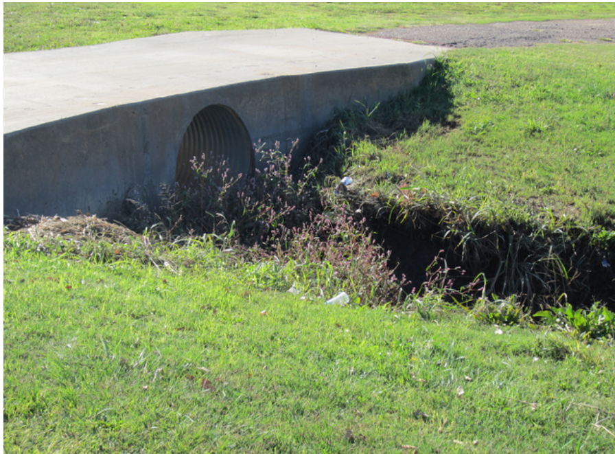
Figure 27: Scouring at Bridge Crossing B
