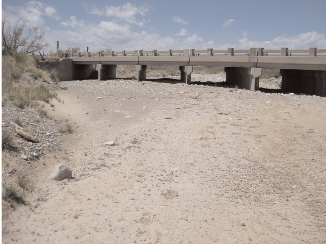
Figure 2.7. Guadalupe Arroyo at upstream crossing of SH 54 looking downstream (larger material in bridge vicinity; bankfull configuration is evident in stream adjacent to this bridge).
