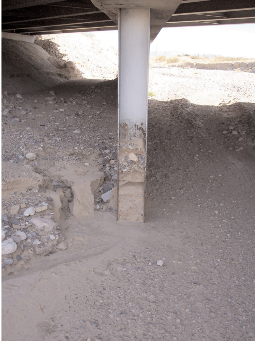
Figure 2.3. Bridge pile (note evidence that bed material has been at least 4 ft higher than it is under conditions at time of the photograph (2009)).(12 in by 12 in steel H piling)
