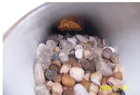
(b) Picture of a circular culvert with sediment deposited for the entire length
