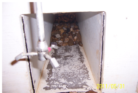
(a) Upstream view through a square culvert showing the development of sediment clogging.
