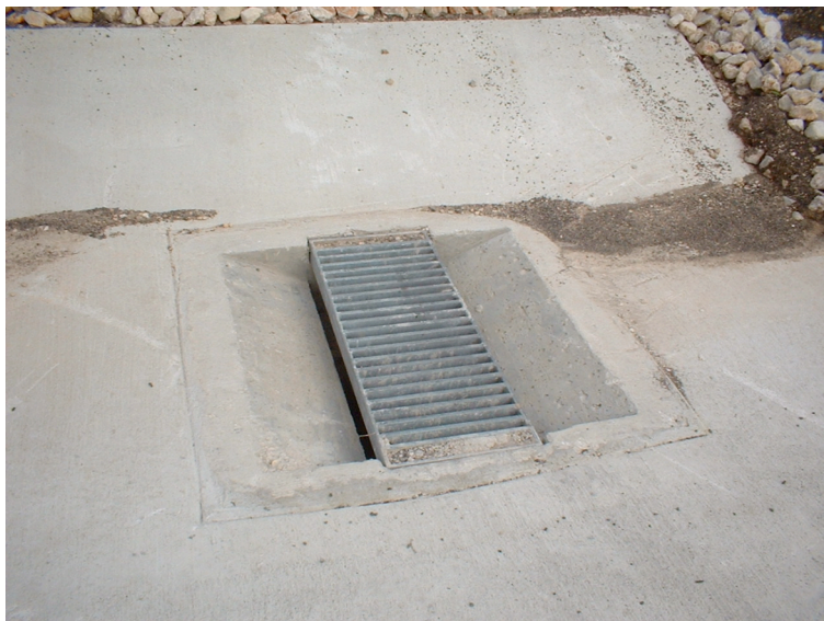
Figure 2. Type-H Inlet (grate top), sloped entry. I-35 feeder near San Marcos, Texas.
