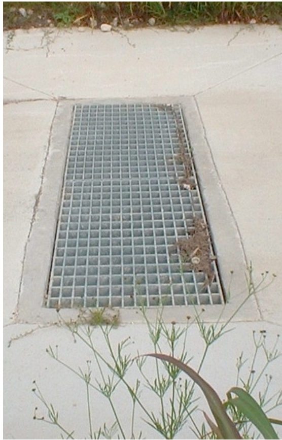
Figure 4. Roadside grate inlet. I-35 feeder near San Marcos, Texas.
