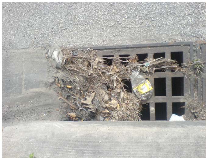
Figure 6. Image of Curb and Grate Inlet with Debris Residue.
