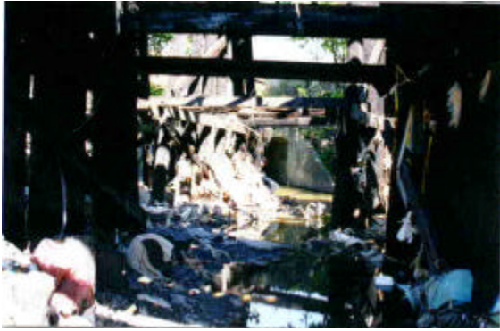
View looking upstream under HB&T RR Bridge. Trash consists of grocery bags, cans, clothing, paper goods, prophylactics, insulin syringes, fiberglass insulation, shoes, yard waste (leaves). March, 1998
