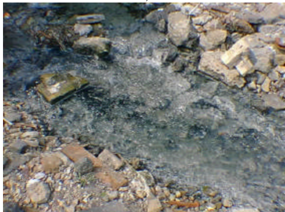
Water in fast-flowing narrow channel beneath RR bridge. Good clarity, black streaks are sediment. May, 1998
