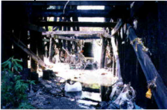
View under RR Bridge showing trash accumulation in piers of bridge. March, 1998
