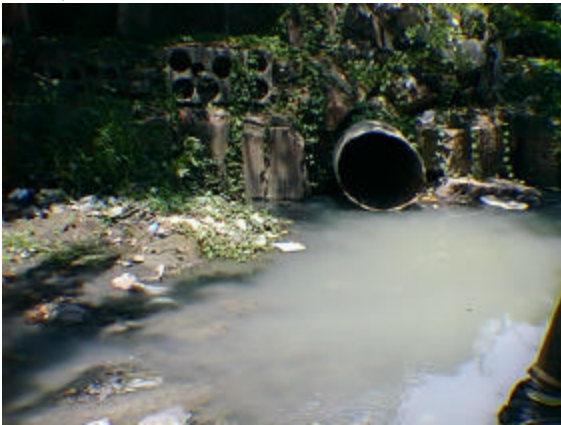
Milky water at culvert June, 1998
