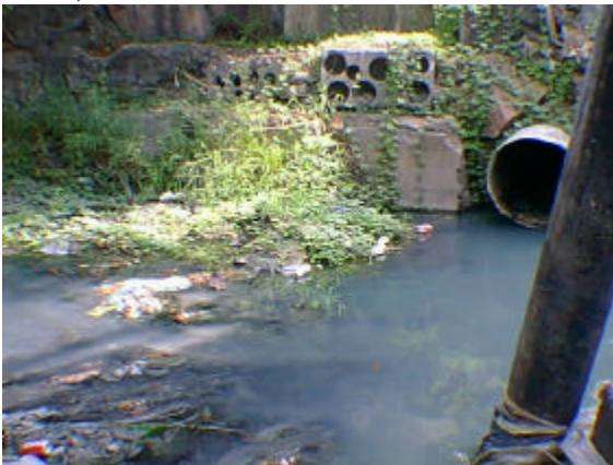
Milky water at culvert August, 1998
