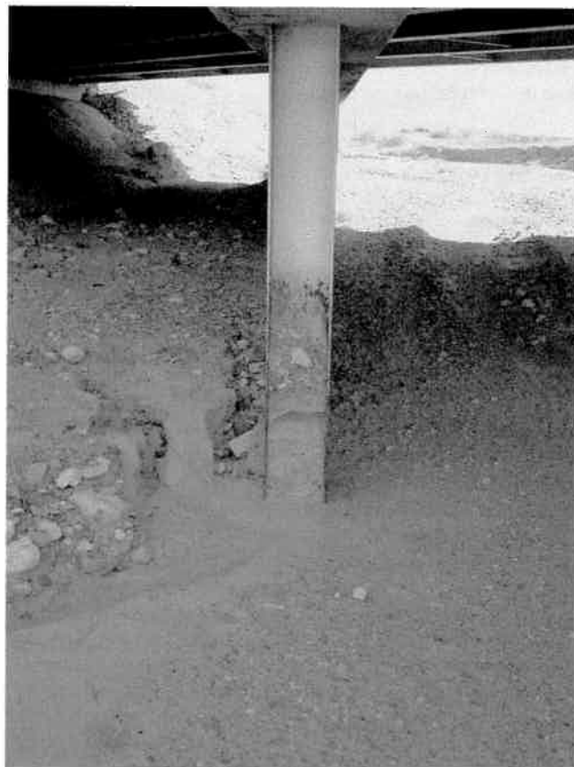
FIGURE 3 Bridge pile (note evidence that bed material has been at least 4 ft higher than it is under conditions at time of the photograph).
