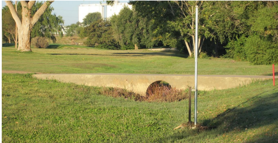
Figure 8: Photograph looking upstream at culvert. Crest gage is vertical pipe in front of the culvert. The golf cart path runs along the top of the culvert
